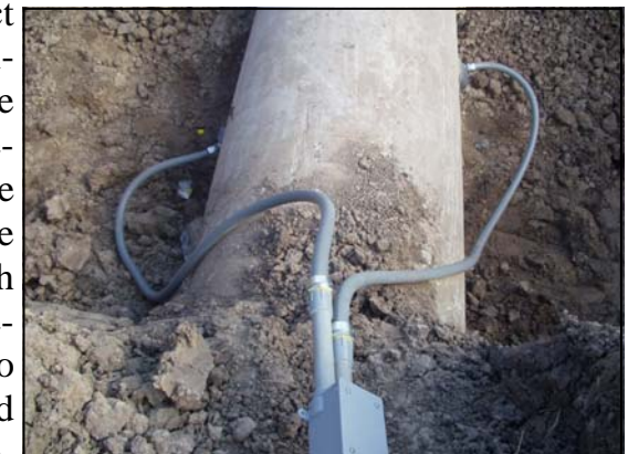
Siemens meter Installed in concrete pipe
