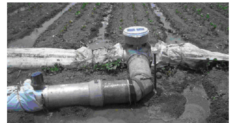
Surge Irrigation Valve (center) and Flow Meter (left)
