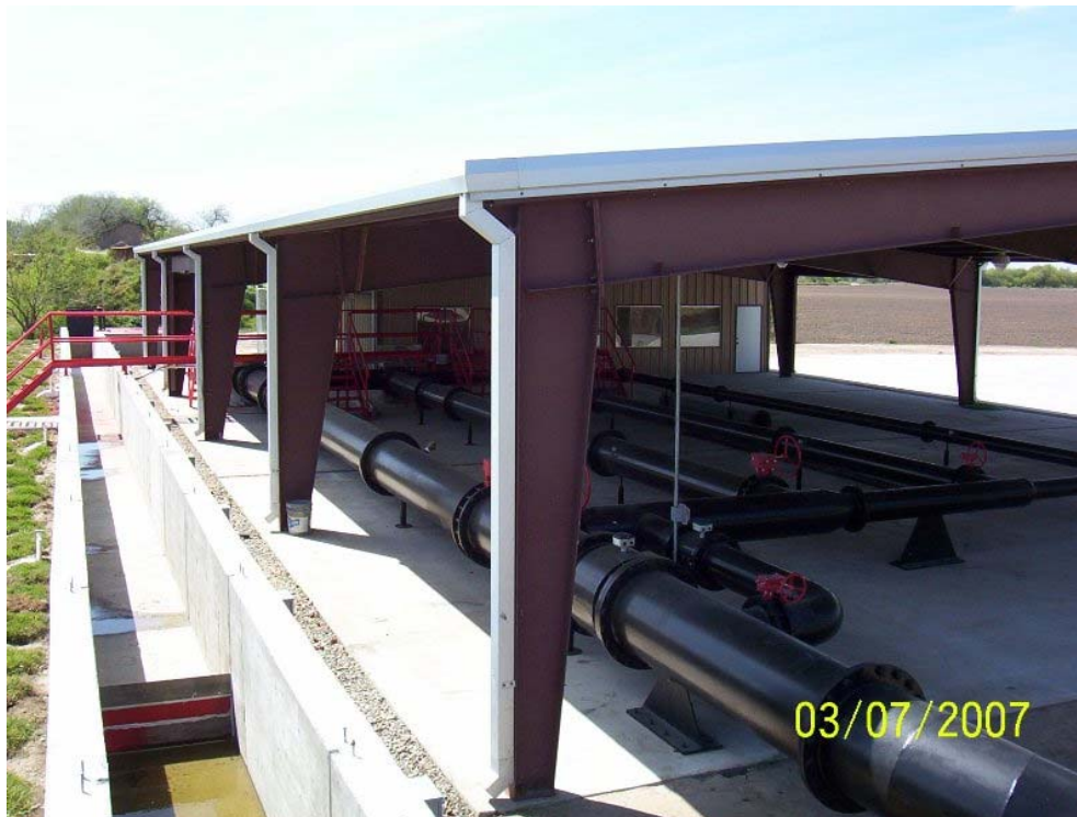
. Figure 2 – Flow Measurement Manifold System
