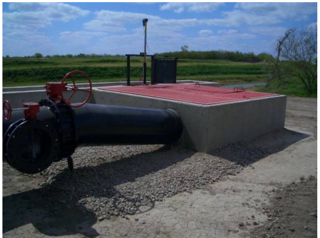
Manifold discharge and calibration tank
